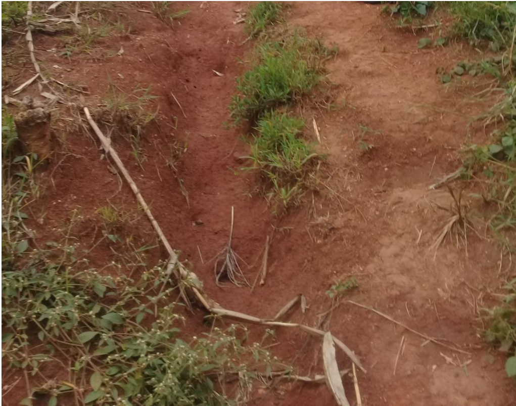
Plate 1: Gully erosion on a deforested steep slope in Kapeeka village Kabango parish Masindi district. Source: Field survey 2017
